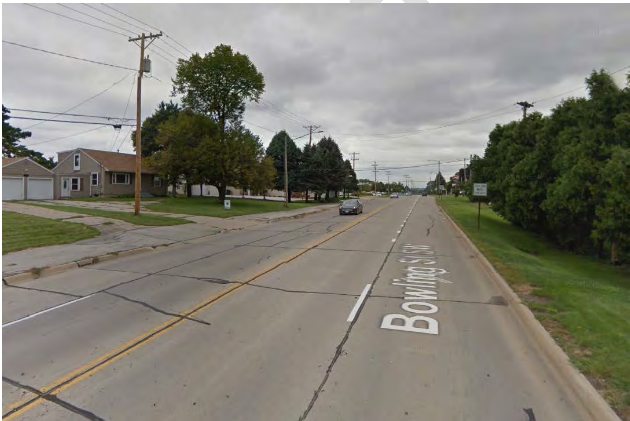
Figure 1 Looking north on Bowling Street SW, between Wilson Avenue SW and 29 th Avenue SW
